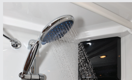
When you're draining down the water system, don't forget the shower head
