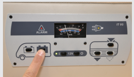
If your battery is only reading 12V, it's flat. A fully charged battery will show at least 12.8V on the panel
