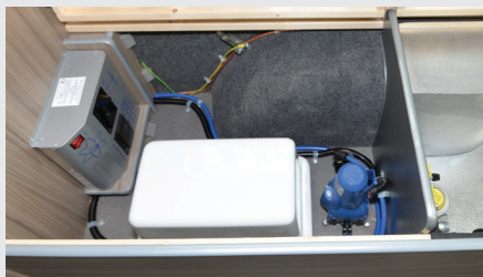
Water pumps (blue device) and hoses need to be drained down over winter
